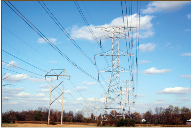
figure 6. Existing 138 and 345 kV transmission lines in rural area near Pendleton, Indiana.
