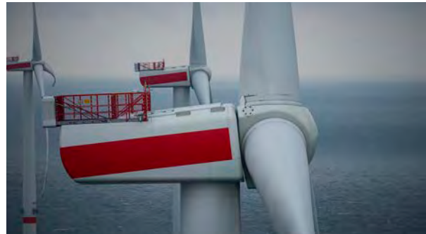
Credit: MHI Vestas Offshore Wind
